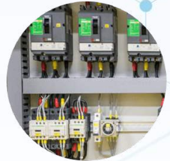
LV Panel Distribution
